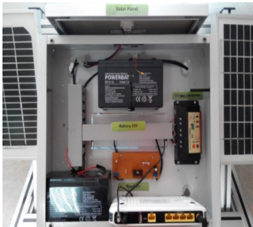
Figure 3: The Prototype of solar powered wireless router
